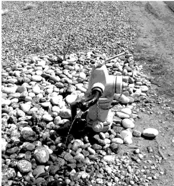
Hydrant flow when the valves were shut.
